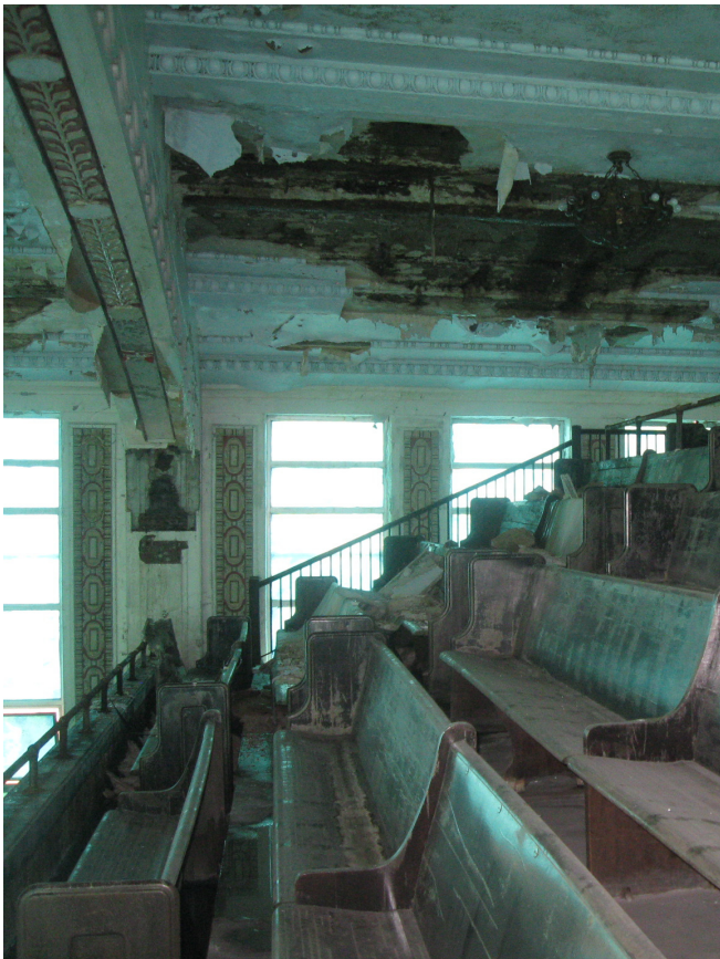
Photo 50. Water damaged pews at balcony
