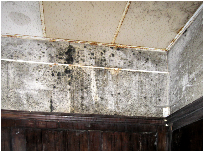
Photo 43. Mold growth on plaster at upper extent of lobby walls
