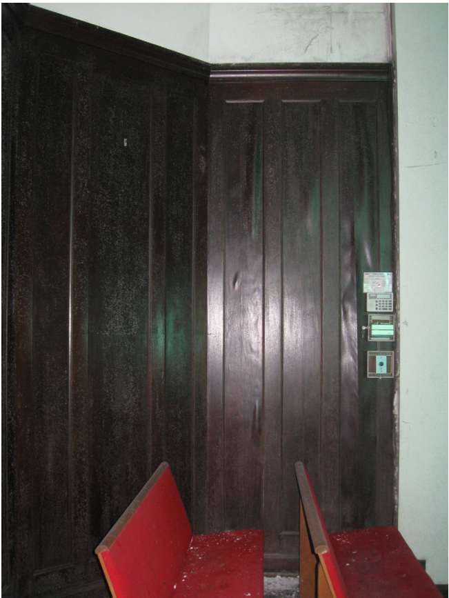
Photo 49. Warped veneer at wood paneling
