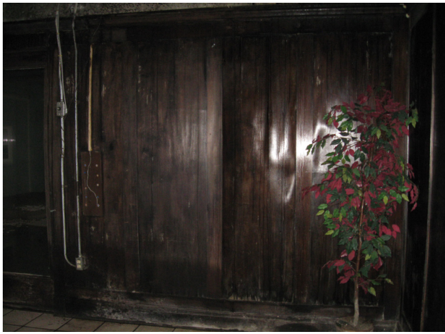
Photo 42. Warped veneer at lobby paneling
