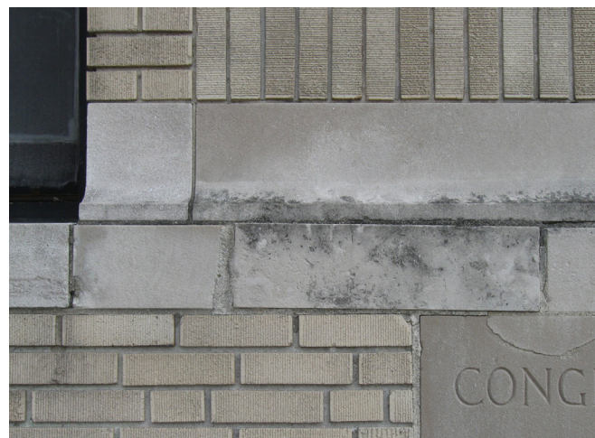
Photo 33. Mortar deterioration at limestone
