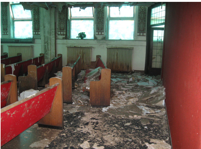
Photo 48. Damaged and mold covered pews
