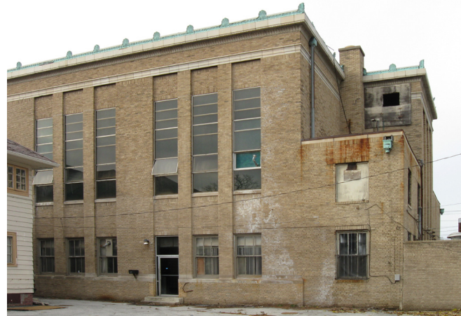
Photo 31. Efflorescence, rust stains, and mortar deterioration at southeast corner
