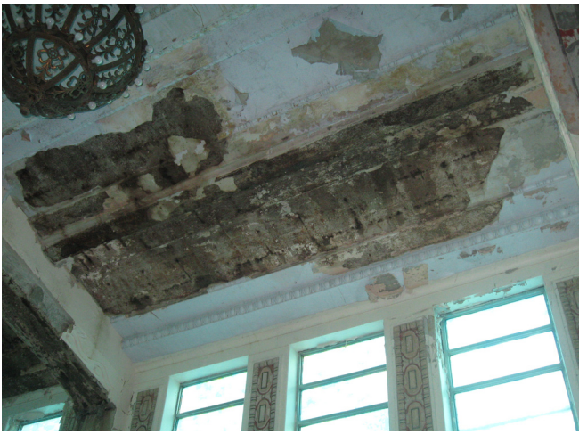
Photo 46. Detail of plaster damage at sanctuary ceiling
