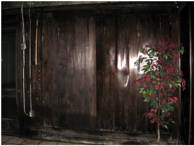
Photo 42. Warped veneer at lobby paneling
