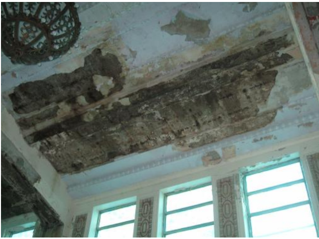
Photo 46. Detail of plaster damage at sanctuary ceiling
