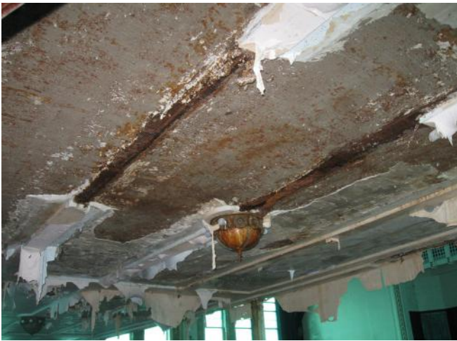
Photo 47. Detail of plaster damage at underside of balcony ceiling
