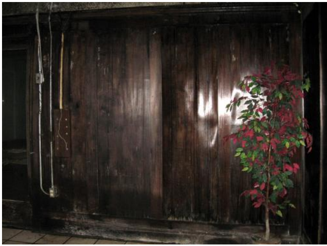
Photo 42. Warped veneer at lobby paneling
