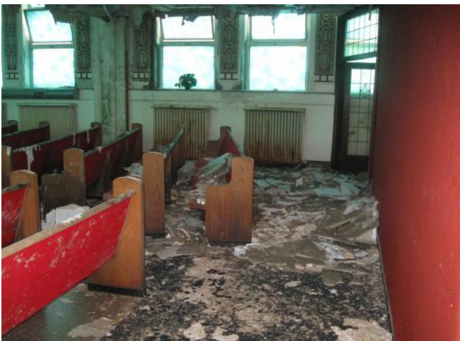
Photo 48. Damaged and mold covered pews
