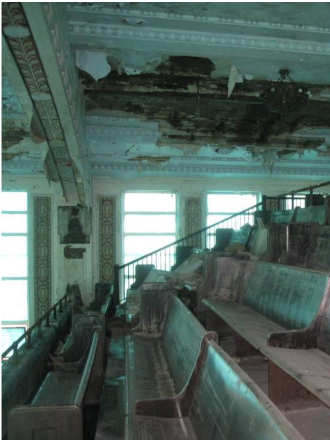
Photo 50. Water damaged pews at balcony
