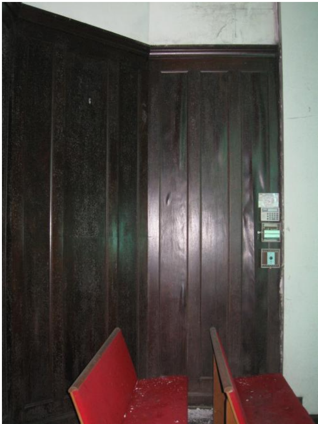
Photo 49. Warped veneer at wood paneling
