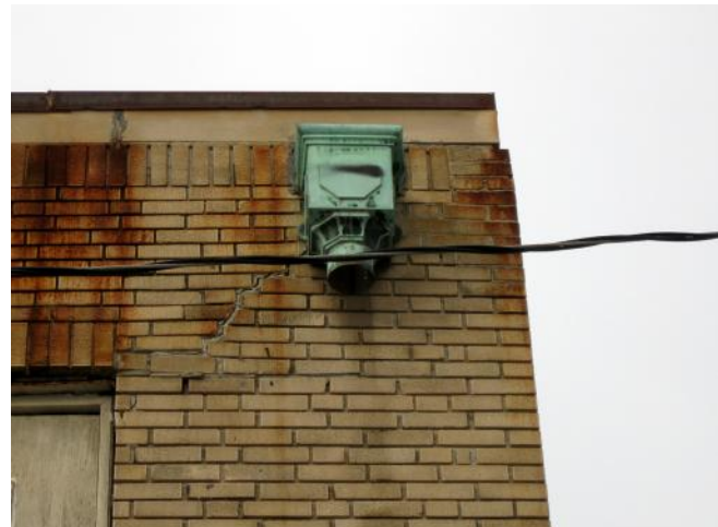
Photo 32. Rust staining, mortar deterioration, and missing downspout at southeast corner
