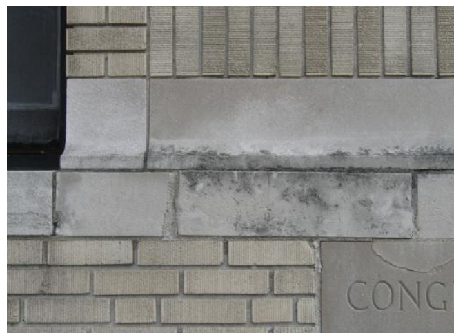
Photo 33. Mortar deterioration at limestone
