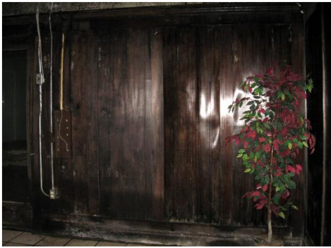
Photo 42. Warped veneer at lobby paneling
